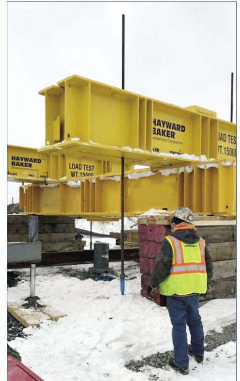
Sensors for this load test include displacement sensor, sister-bar strain gauges, settlement sensors, pressure cells, and piezometers.
