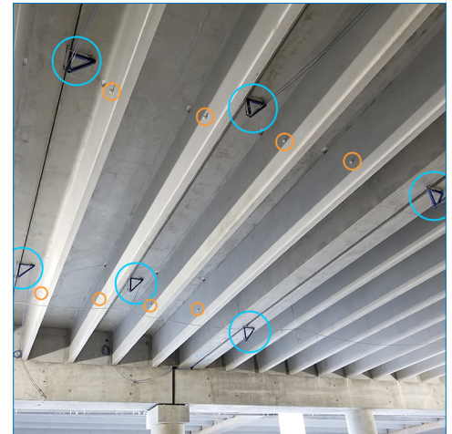
Jointmeters (blue) and wireless tiltmeters (orange) monitoring displacements and twist.
