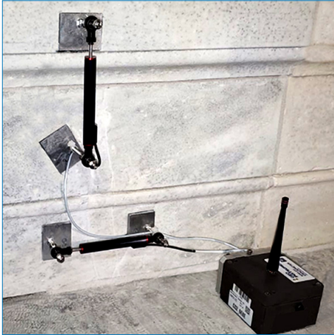
Two crackmeters connected to a GeoCloud wireless crackmeter node.
