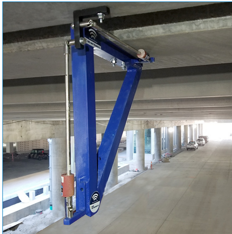
A two-axis jointmeter used to monitor vertical and horizontal movement.
