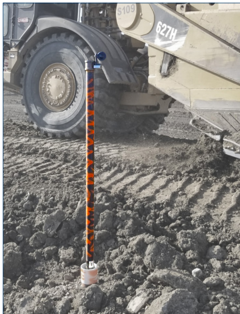
Settlement plate risers should be painted and flagged to be visible to equipment operators.
