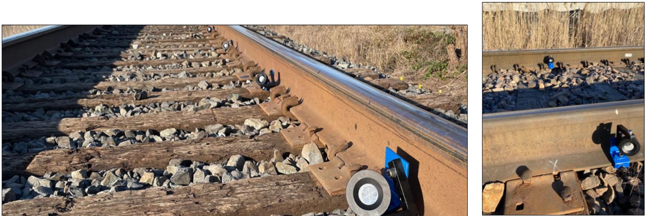
Figure 3: Image of Rail Clip Prisms attached to rails with timber crossies.
