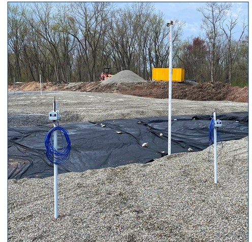
Wireless nodes above are connected to piezometer cables. Prism is attached to the top of the settlement plate riser.
