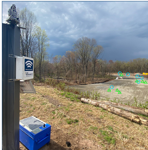
AMTS and co-located gateway are monitoring distant settlement plates and piezometers during ground improvements to a warehouse access road.
