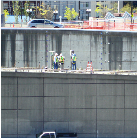
I-5 retaining walls were monitored as a TBM drove through their foundations.
