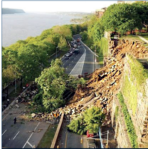
Multi-year monitoring was required for repair of this massive wall failure.
