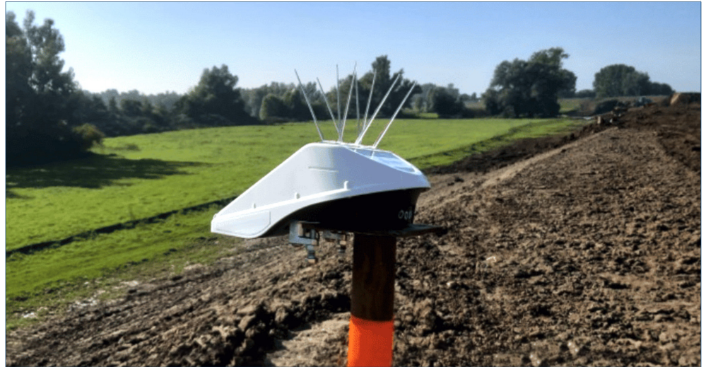
Locator One sensor mounted on settlement plate riser pipe and protected by bird spikes
