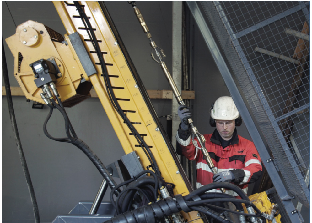
DeviGyro ready for a survey
