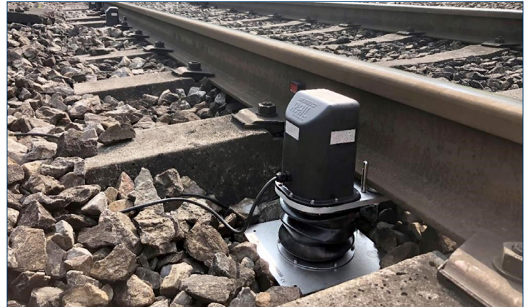
FLX-Rail sensor records the maximum deflection of dynamically loaded track
