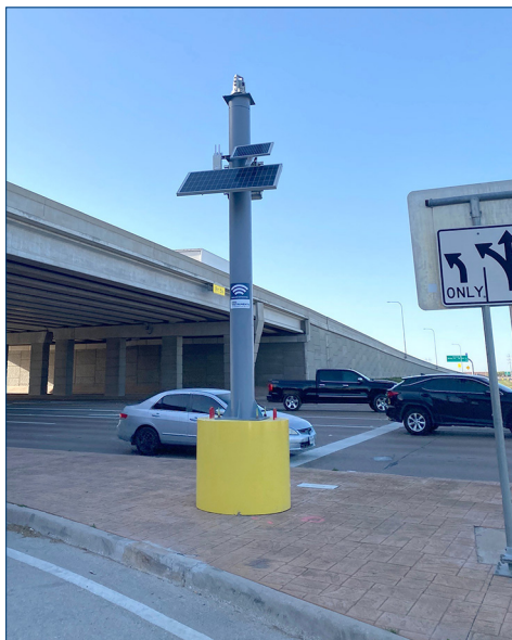
Towers can be located nearly anywhere
