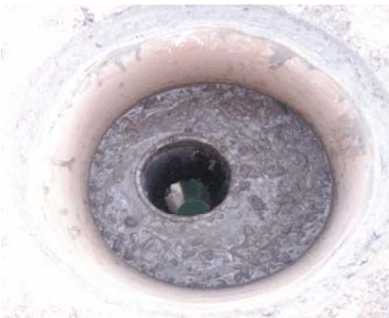
Left:: Cored hole in pier pavement to accept the flush mounted logger system.
